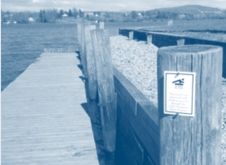
A dock installation in Ticonderoga was funded by a LCBP Public Access grant.
