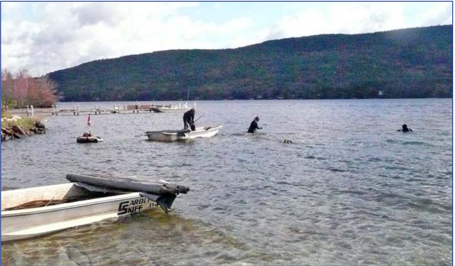
Contracted dive crews install benthic barrier mats at Lake Avenue. Photo courtesy of Lake George Association
