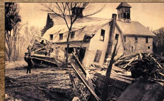
After many years of use, the barn and garage gave way to bulldozers in May 1975, making space for the Ledgewood development.
