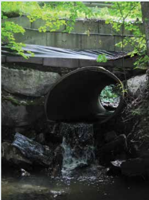
This undersized and "perched" culvert blocked passage of aquatic organisms such as fish.
