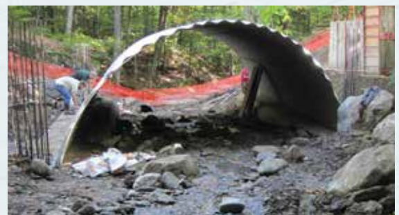
This open bottom culvert allows stream flow and aquatic organism passage (note people working by huge culvert).
