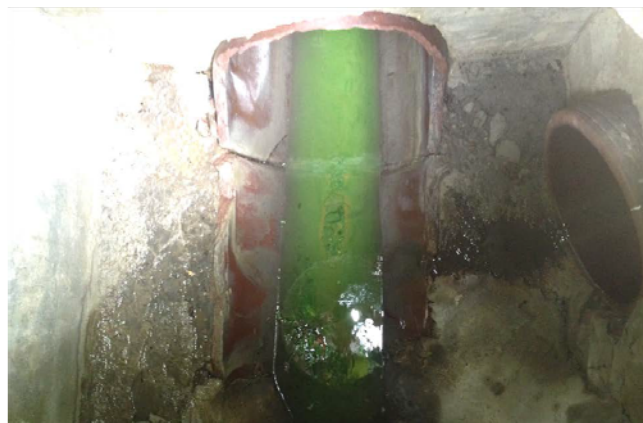
Dye testing of toilets in two houses on North Pleasant Street in Middlebury revealed cross connections to a stormwater line, visible in
