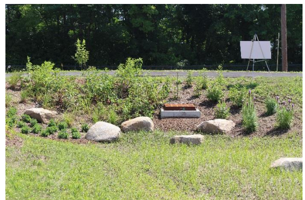
Figure 5-18. Photo of bioretention basin outlet
