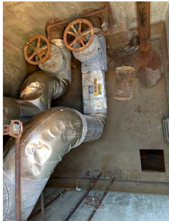
Figure 4. HVAC vault adjacent to PB03 stormdrain
