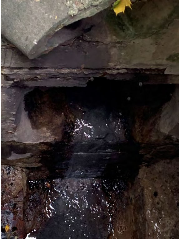
Figure 12. Wastewater in stormdrain on Couch Street
