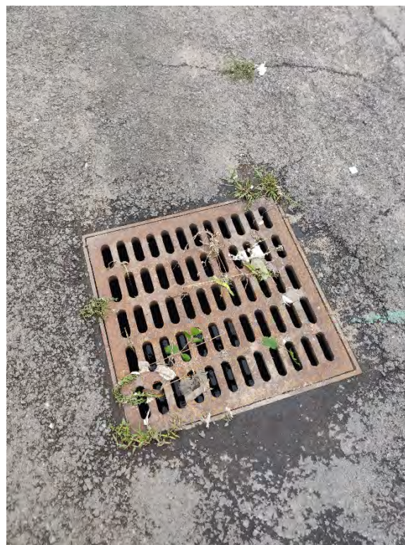
Figure 11. Toilet paper on catchbasin CB01 grate following sewer overflow event
