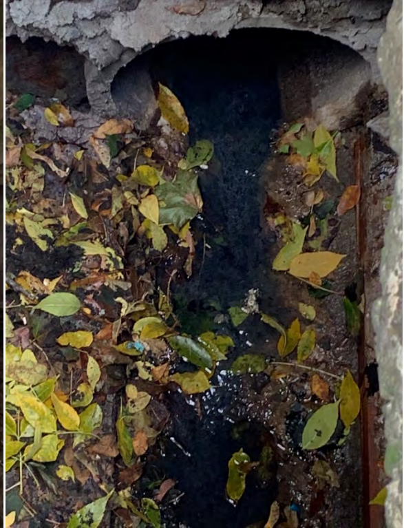
Figure 13. Wastewater in stormdrain at the intersection of Brinkerhoff and Helen Streets
