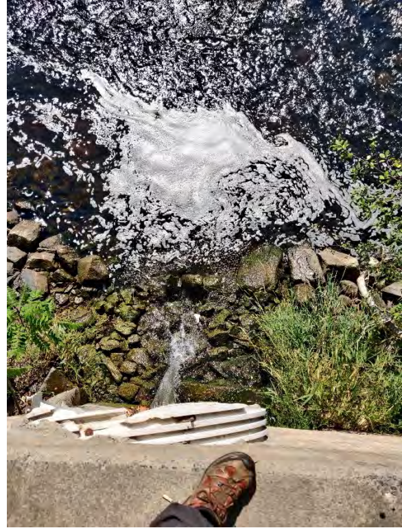
Figure 3. Suds at the outfall of PB03 in July 2020
