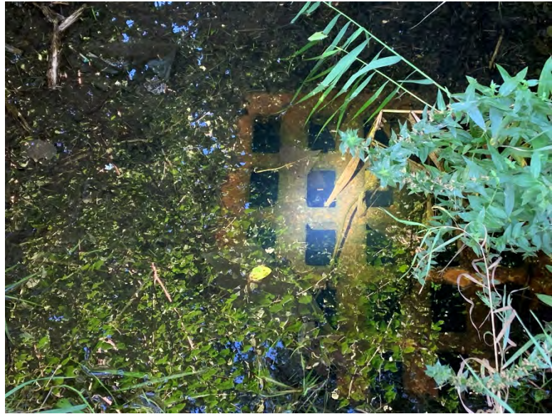
Figure 18. Flooded catchbasin CB01
