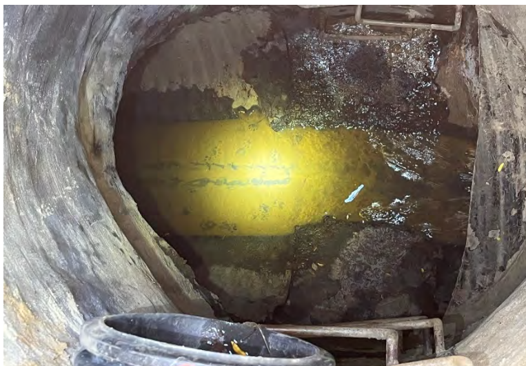
Figure 9. Tracks in manhole MH02.
