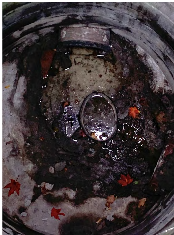
Figure 5. Catchbasin CB01 in the PB04 stormdrain
