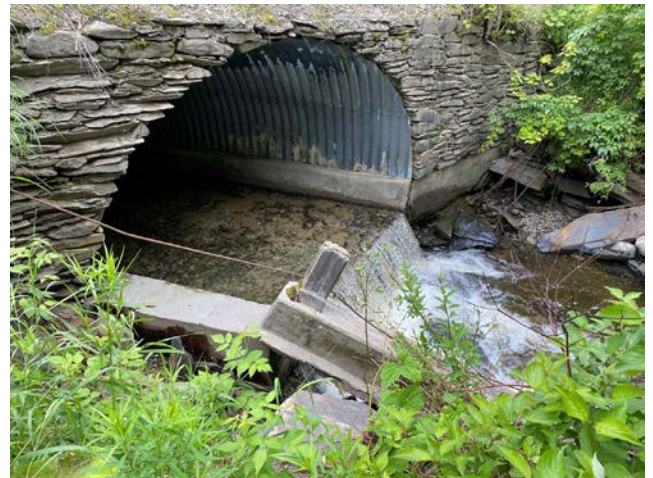
Perched culvert on Stannard Brook at intersection of Stannard Mtn Road and Lazy Mill Rd in Stannard, Vermont
