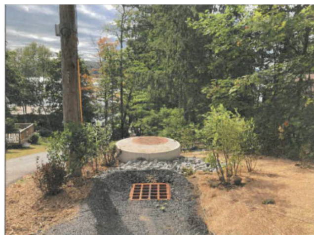
A hydrodynamic stormwater separator installed in 2021 as part of phase one of the upper Trinity Rock Road storm sewershed.
